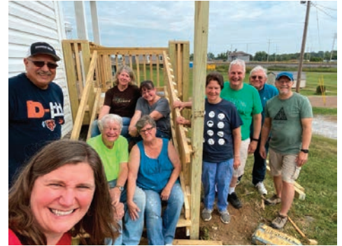
FCC Paducah joined other Fuller Center volunteers to build a new home on a site impacted by the 2021 tornado in Mayfield.
